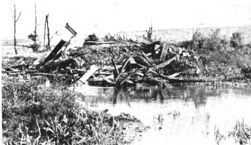
DEMOLISHED BRIDGE, OLD FORGES CONSENVOYE ROAD
